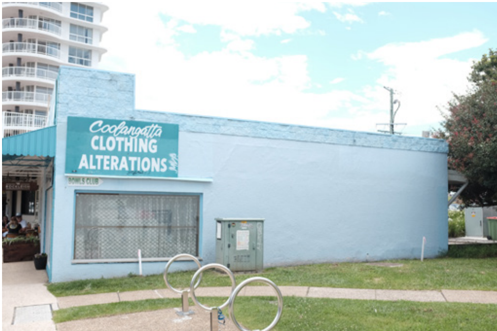
[LEFT] Mural 1 : Width: 9 m, Height: 3 m NBN Cabinet size: Width 1m, Height 1.2m, Depth 0.55m
